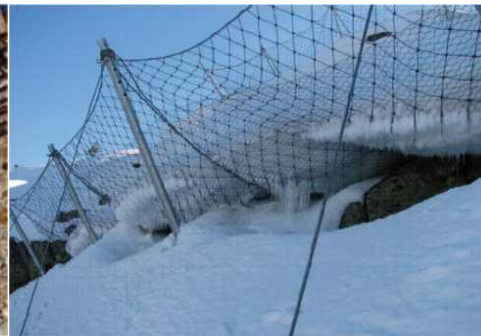
Fig. 6(b). Guywires, snow cable nets
