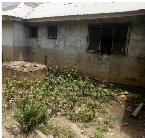
Plate 3. Flood mark on wall depicting the maximum flood depth in Ogbaru
