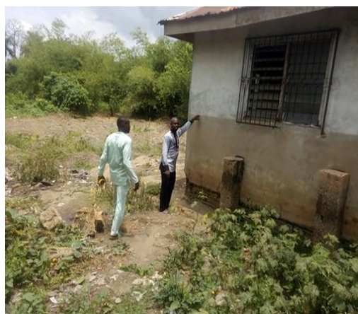
Plate 2. Flood mark on wall depicting the maximum flood depth in Ogbaru
