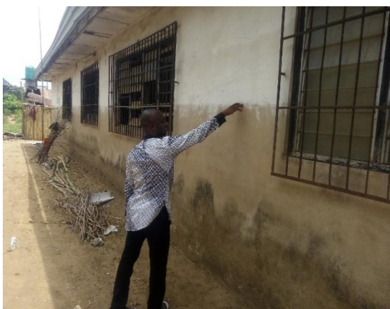
Plate 1. Flood mark on wall depicting the maximum flood depth in Ogbaru
